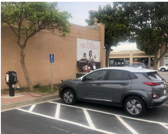
FIGURE 35: LEVEL 2 EVSE IN DOWNTOWN GUADALUPE (PHOTO: PLUGSHARE)
