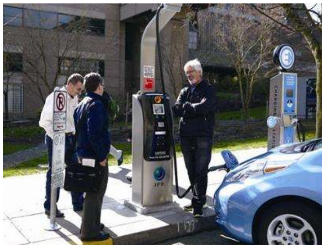
Figure 15: RAPIDAS / Kanematsu 208 volt Battery Backed Fast Charger on Portland’s “Electric Avenue” 17
