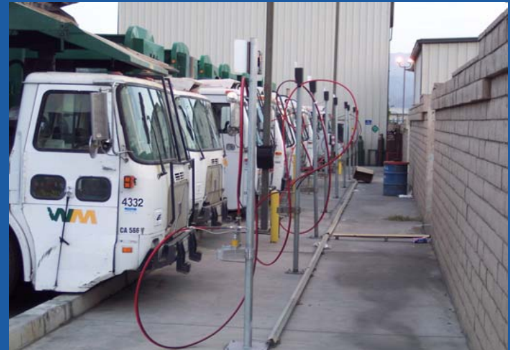
Waste Management CNG Time-Fill Station
